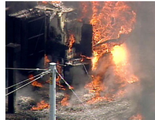
Lakeland FL, August 2007. Ignition of 14 000 gallons of oil!
