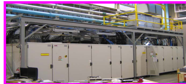
10 MW Converter "Amplifier"
