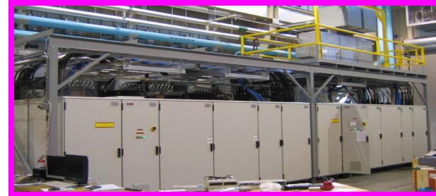
5 MW Converter "Amplifier"
