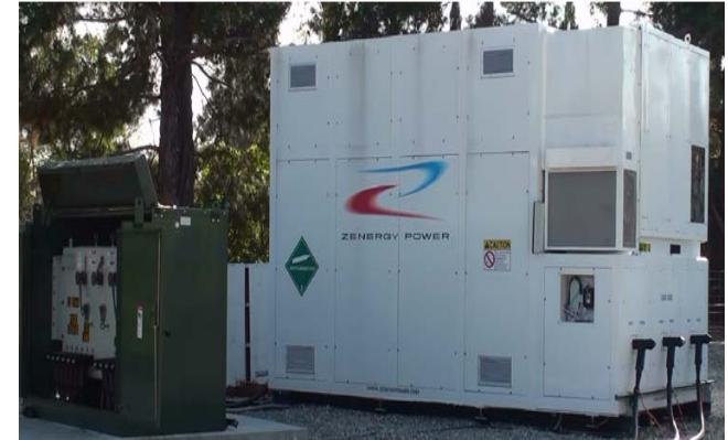
Initial Zenergy FCL Installation on SCE Grid
