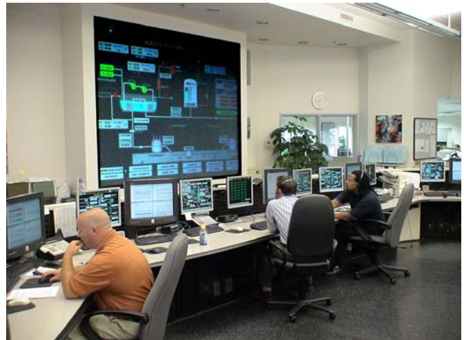
Fig. 3. Remote Operations Center. Albany HTS cable system is monitored from the BOC facility in Bethlehem, PA.
