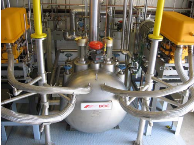
Fig. 1. Cryogenic Refrigeration System. Hybrid refrigeration arrangement using interchangeable cryocoolers and back-up liquid nitrogen.
